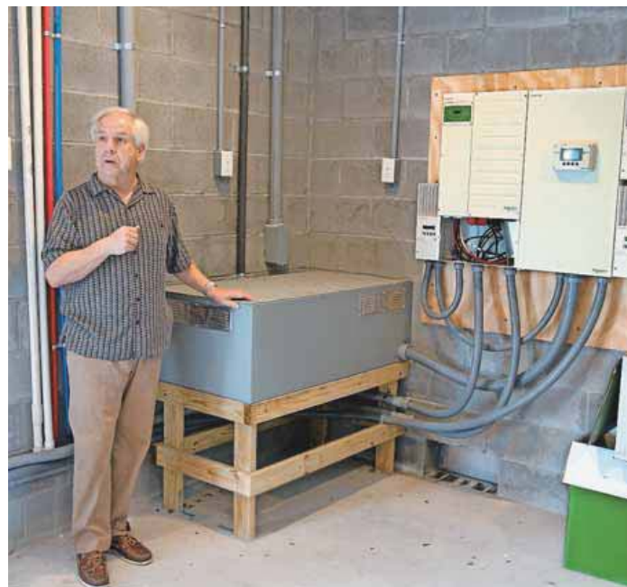
Steve Bostic, managing partner of Amerisips, shows a state-of-the-art standby 50 amp solar power system utilizing lithium-ion batteries that operate "off the grid."
