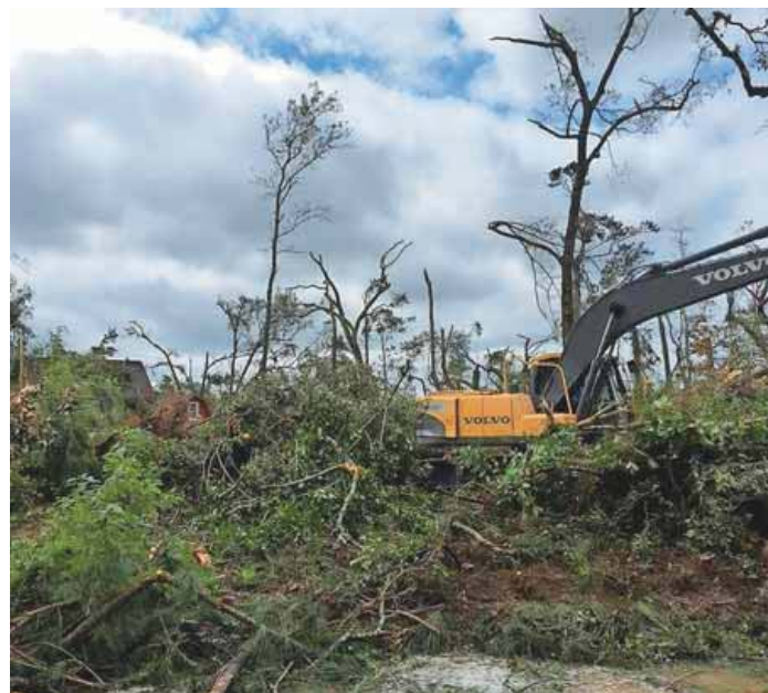
Work crews man bulldozers and backhoes to clear out fallen trees on Sonny Boy Lane on Johns Island, hit by a tornado two weeks ago.
